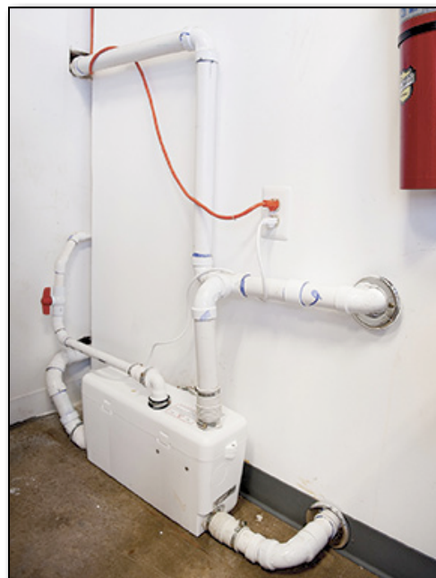
SCHMACHER & SEILER CHOSE TO INSTALL THE SANIBEST MACERATOR BEHIND THE RESTROOM WALL, SO THAT IT IS NOT VISIBLE. EFFLUENT IS PUMPED FROM THE UNIT THROUGH SMALL-DIAMETER PLASTIC PIPING.
