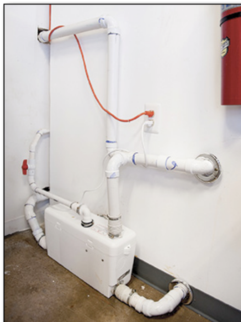
SCHMACHER & SEILER CHOSE TO INSTALL THE SANIBEST MACERATOR BEHIND THE RESTROOM WALL, SO THAT IT IS NOT VISIBLE. EFFLUENT IS PUMPED FROM THE UNIT THROUGH SMALL-DIAMETER PLASTIC PIPING.
