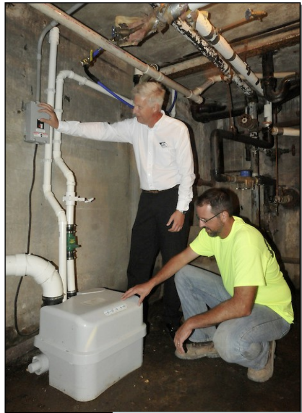
Don Smith of Irr Supply (left) with Scott Kuhns of RIC Plumbing of Lockport, N.Y. Although it was his first Sanicubic installation, Kuhns finished his work in just one day. "This pump is well-suited for the application. The building is very old and digging would have been very difficult."
