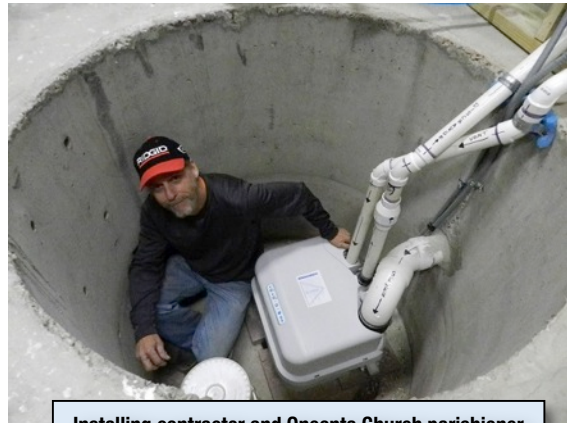
Installing contractor and Oneonta Church parishioner John Stewart with the installed Sanicubic 2 grinding system from Saniflo, which will handle all of the church expansion’s plumbing needs.
