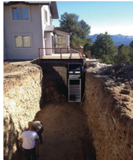
A Rising S underground bunker, which can be used as shelter against natural disasters and widespread civil unrest.
