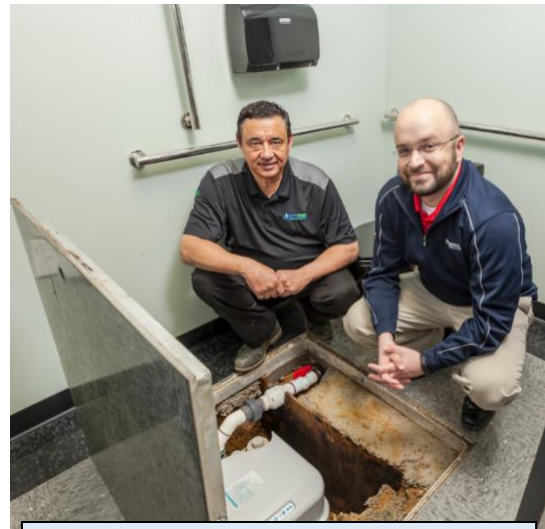
Dale Nichols of PipeTech Plumbing Technologies (left) and Nathan Smith, Ferguson Branch Manager in Raleigh, stand over the Sanicubic 2 duplex grinding system from Saniflo, which grinds and pumps effluent to the drain line.
